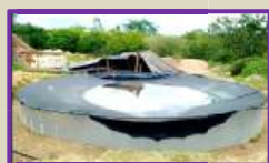
100,000 Litre Water Tank
