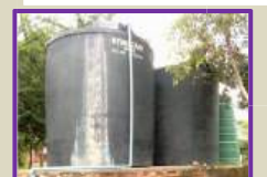
Reserve Water Tanks
