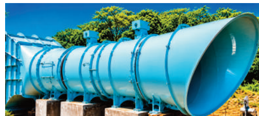
MAIN VENTILATOR FANS
